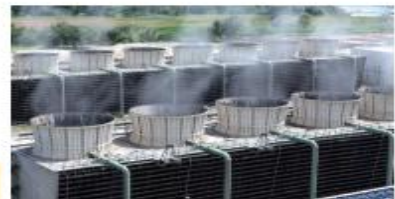
Cooling Tower Energy Saving
